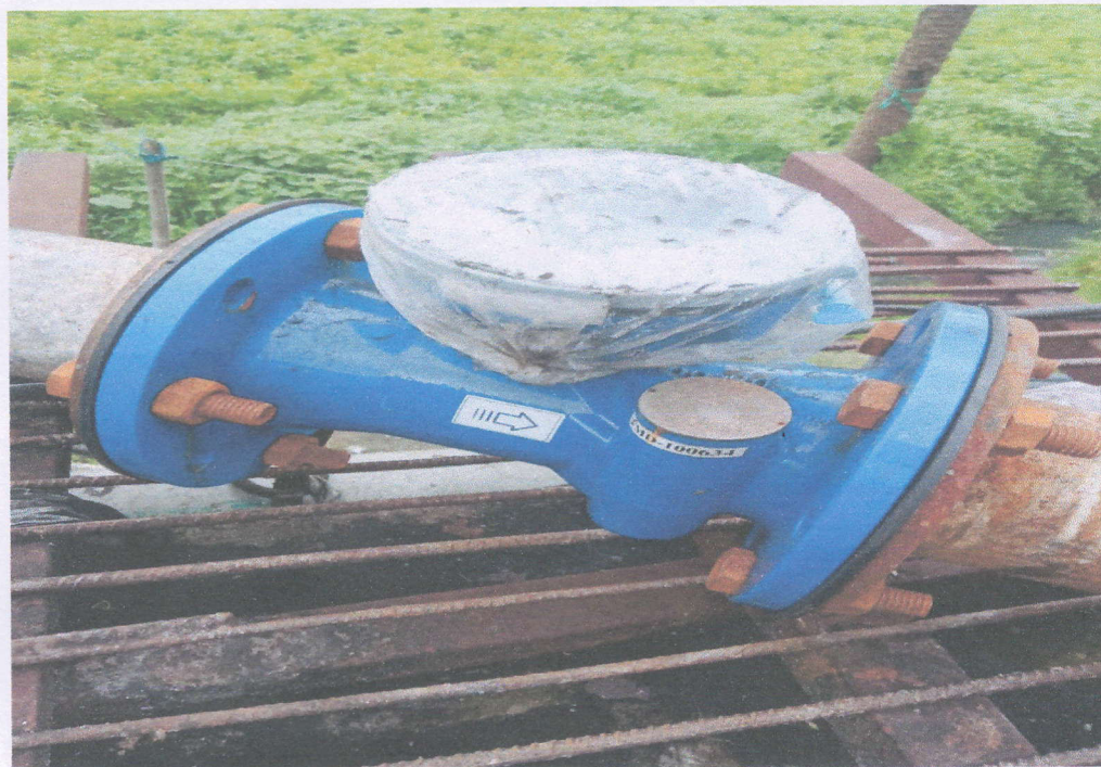
RO Receiver Flow Meter - Factory
