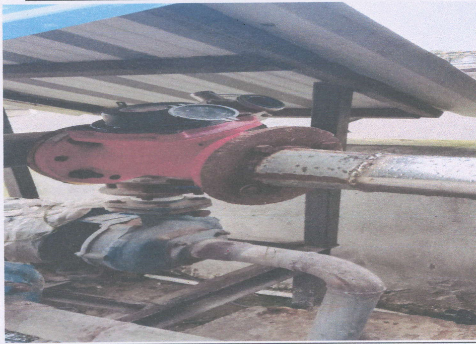
RO Discharge Flow Meter - ETP
